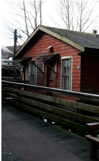
In 2011, the south facade retains its original shingle siding, classic double-hung windows and entry shed roofs.
