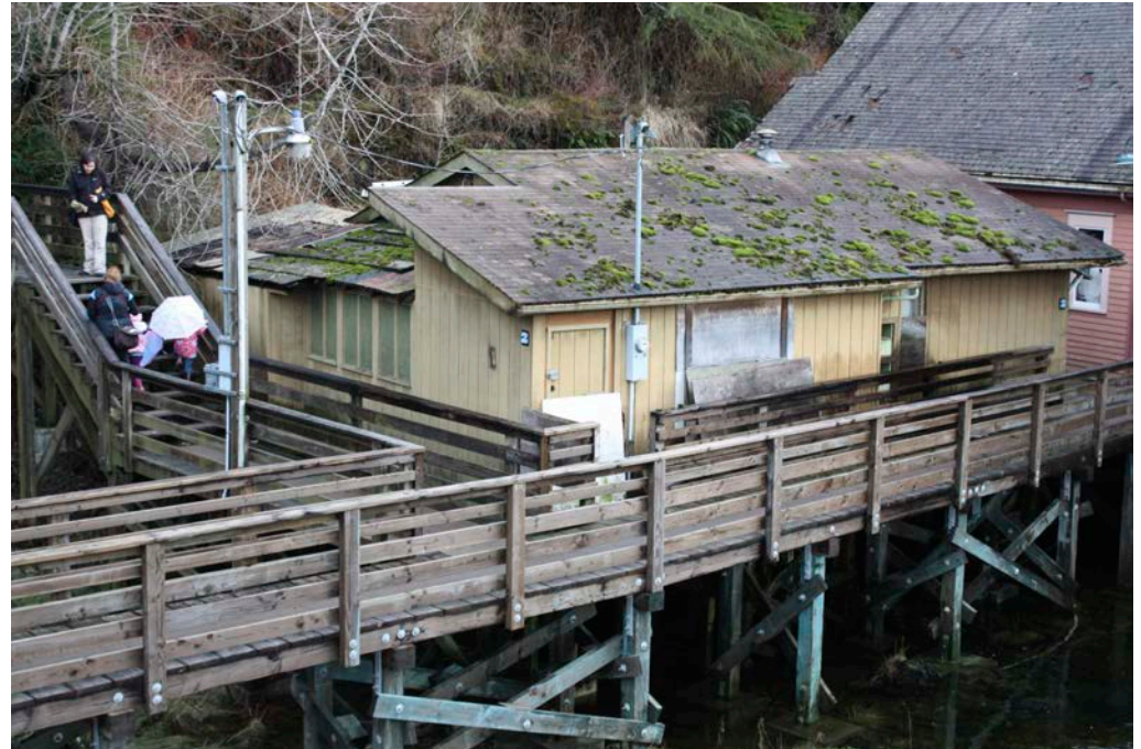
These two primary elevations no longer have period windows and siding (2011 photo). The building is not presently occupied and is in danger of demolition. The City replaced the adjacent boardwalk, railings and piling in 2010.
