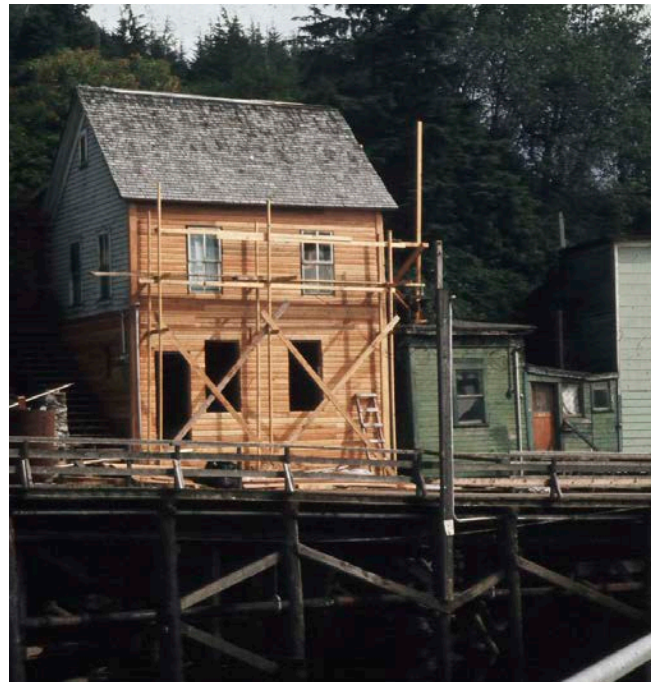
New, locally-milled cedar (Ben Fleenor’s Herring Bay Lumber) to match original siding was needed to repair deterioration on one facade, 1975. Original windows and trim were also restored.
